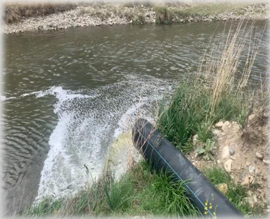
Effluent discharged from 1.75 MLD in river in Location 2, Babesa
